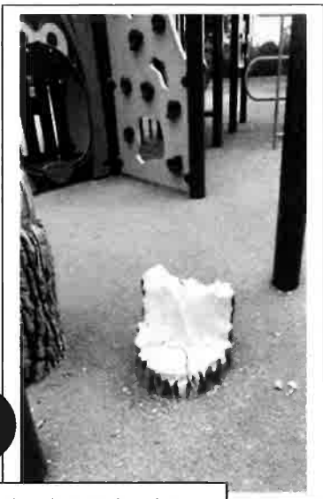
Concrete stump broken
