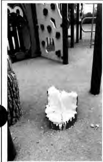
Concrete stump broken
